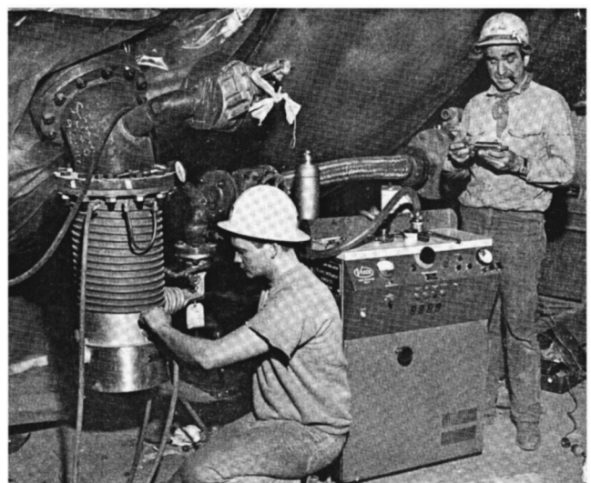
FIG. 6. The entire tank was vacuum leak-tested by Chicago Bridge and Iron engineers. A small mass spectrometer capable of sensitive detection was connected to the vacuum pump and helium was introduced around the tank and all the plumbing. From Sharp Bits , September 1966.
